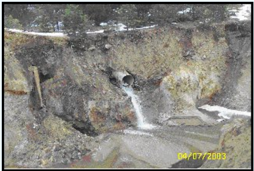
Photo 2: Direct flow path of Balarat Gulch into mine workings under existing conditions
